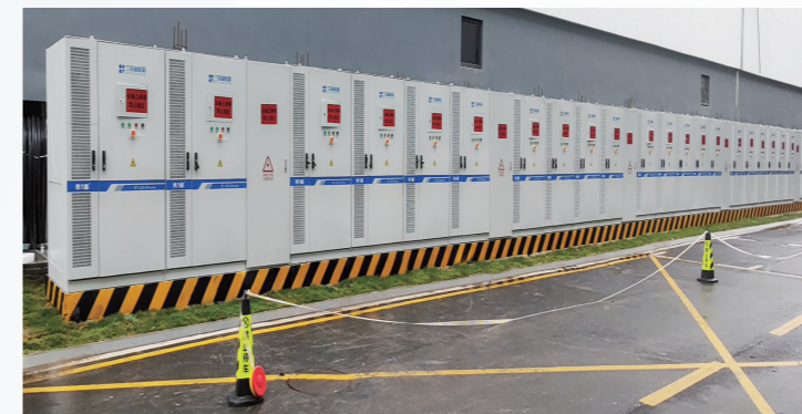
42 x 100 kW/232 kWh energy storage system project in the factory of Shanghai
