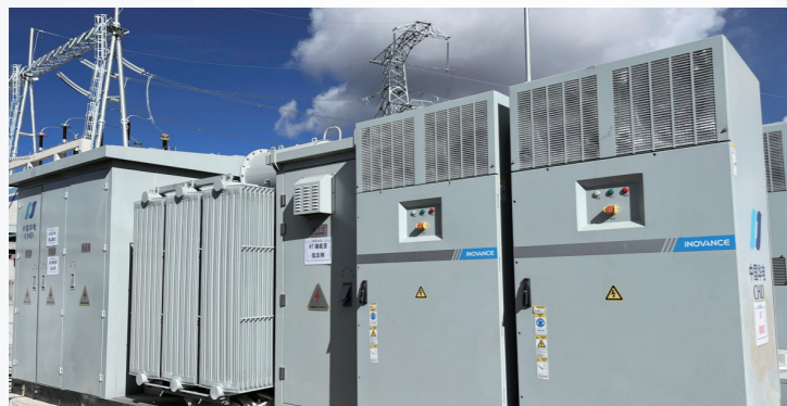
50 MW/50 MWh, photovoltaics, with high-altitude of 4500 m in Yajiang, Sichuan
