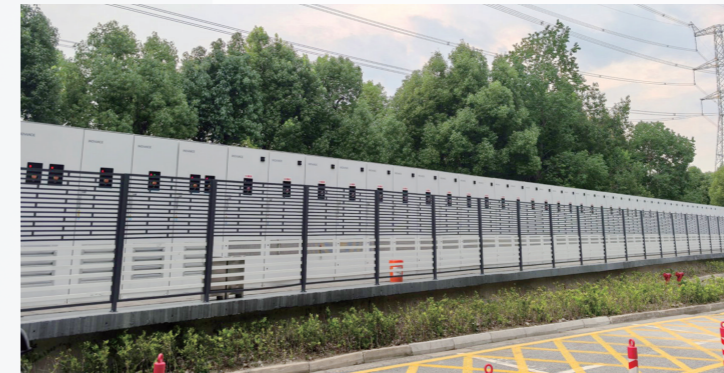
37 x 125 kW/261 kWh energy storage system project in the factory in Suzhou, Jiangsu
