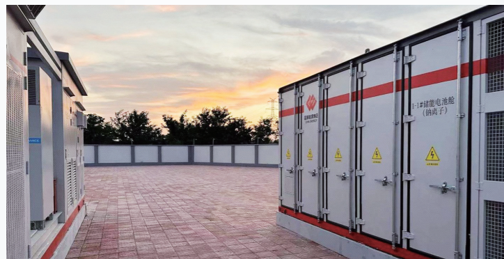
Sodium-ion battery- 150 MW project in Penglai, Shandong
