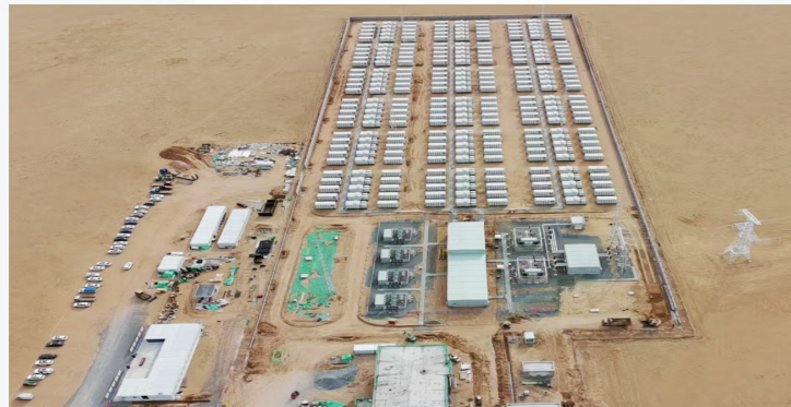
450 MW/900 MWh, power station, in Inner Mongolia
