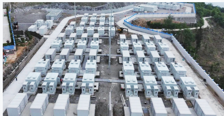
100MW/200MWh grid-forming project in Mulipo, Yunnan
