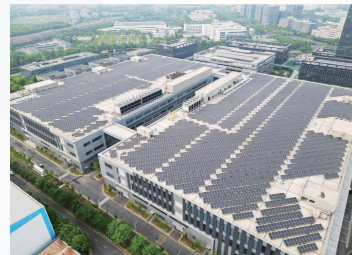
1MW/2.08MWh integrated optical storage and charging project in the factory of Nanjing, Jiangsu
